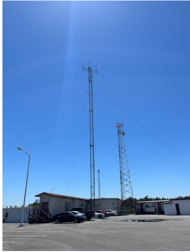
Figure 45: RRU Tower at Pinecastle Range
