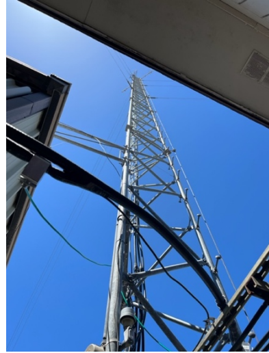
Figure 46: Equipment on RRU Tower
